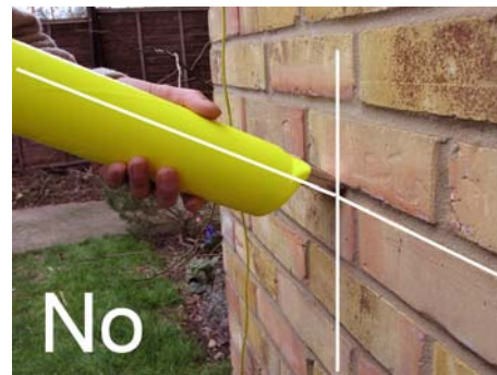
Nozzle is incorrectly seated in the mortar joint
